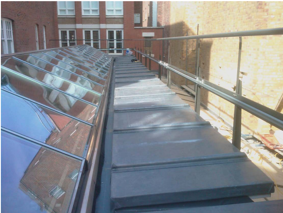
Unirail lifeline fitted to the balustrade.
