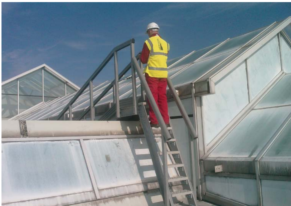
Fibreglass anti-slip textured access steps allowed access over the north light roofs.
