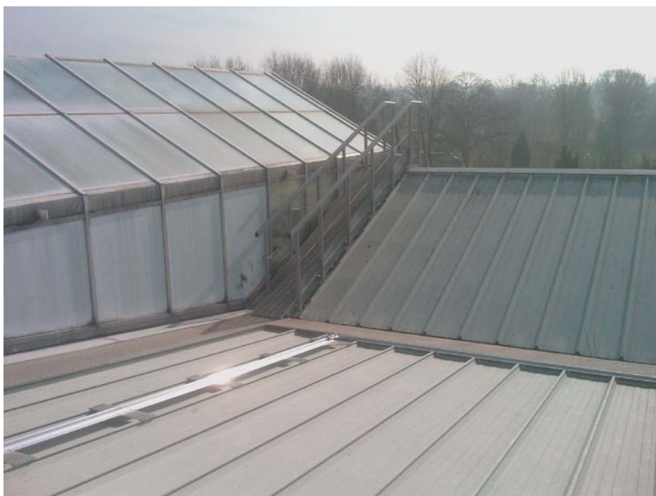
Fibreglass anti-slip textured walkways provided a safe surface to walk on and protected the roof sheets from footfall damage.
