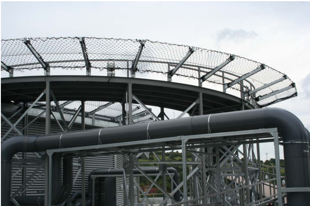
The curved ramp section had to accommodate changes to the clients design at the 11 th hour.
