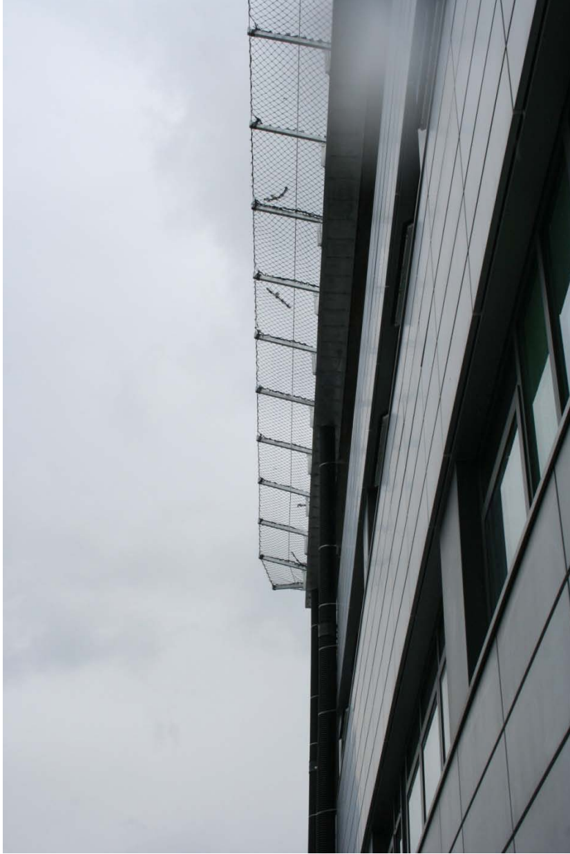
On some sides the drop was 30m with tight space below making roped access ideal.
