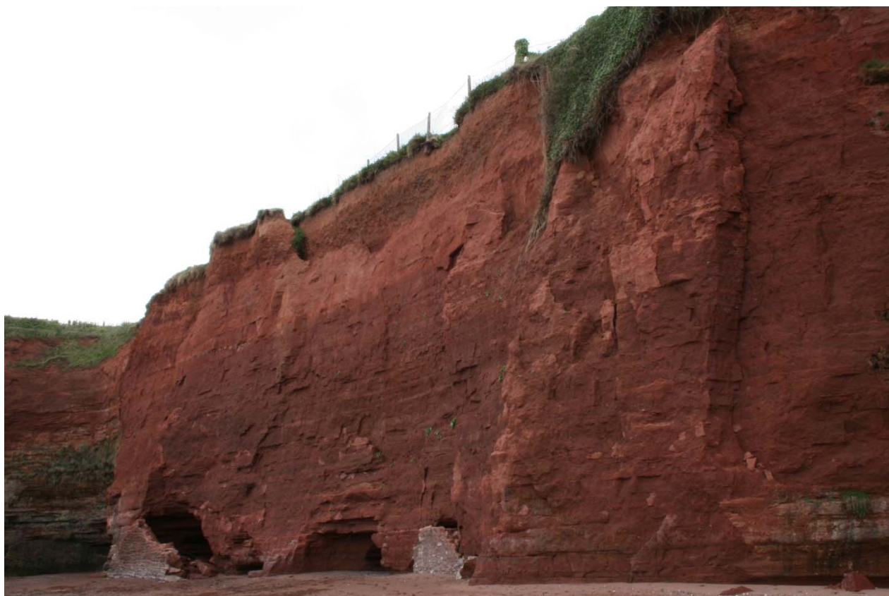
Hollicombe bay cliffs prior to remedial works
