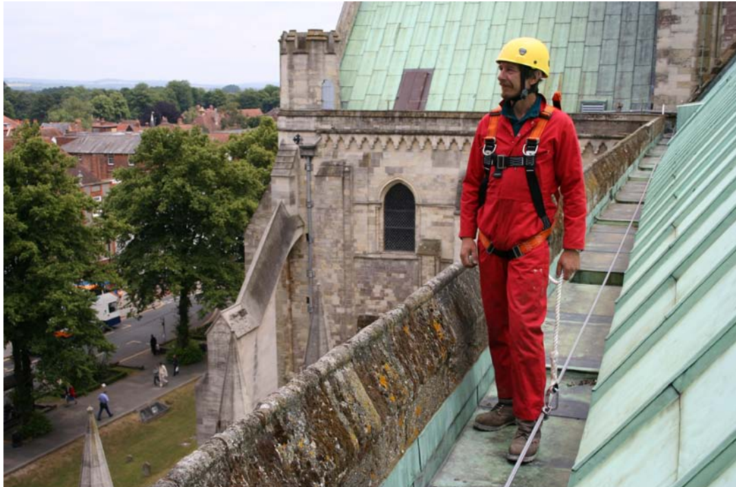
Grey coloured Uni16 synthetic lifeline fitted to the Nave roof, Chichester Cathedral.
